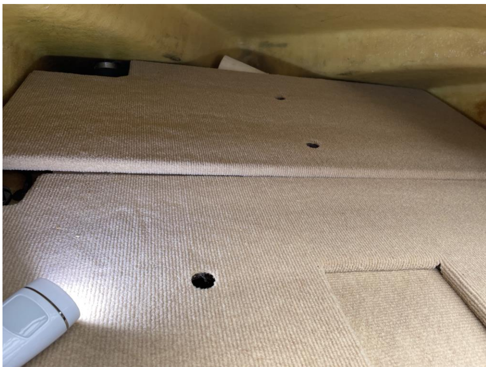
Both boards fitted (The angle of the photo makes it look distorted but it isn't).
